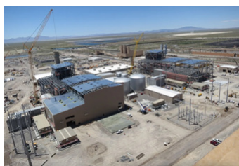
Construction of two hydrogen-capable natural gas generators proceeds at the IPP site in July 2024.
